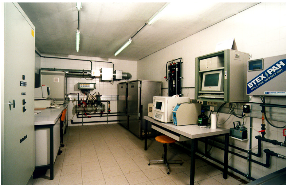
Figure 7: Online - monitoring station for water quality
